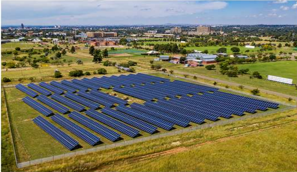
The solar plant on the UFS's Bloemfontein Campus, part of the university's commitment to combatting loadshedding and embracing sustainable energy.
