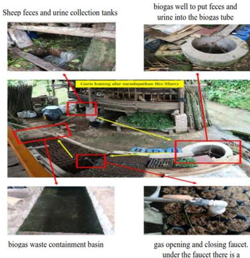
Figure 3. Digester Installation for BIOS+ Product Manufacture
