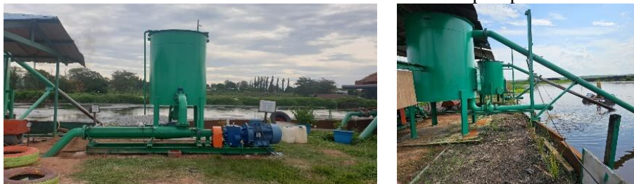
Figure 4. Position of the PCP Pump and the Vertical Vacuum Filter Tank
