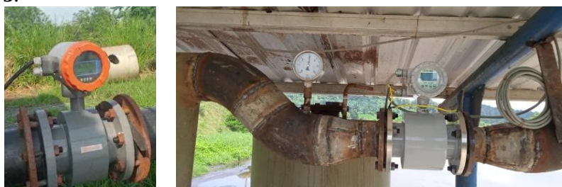
Figure 5. Flowmeter and Pressure gauge
