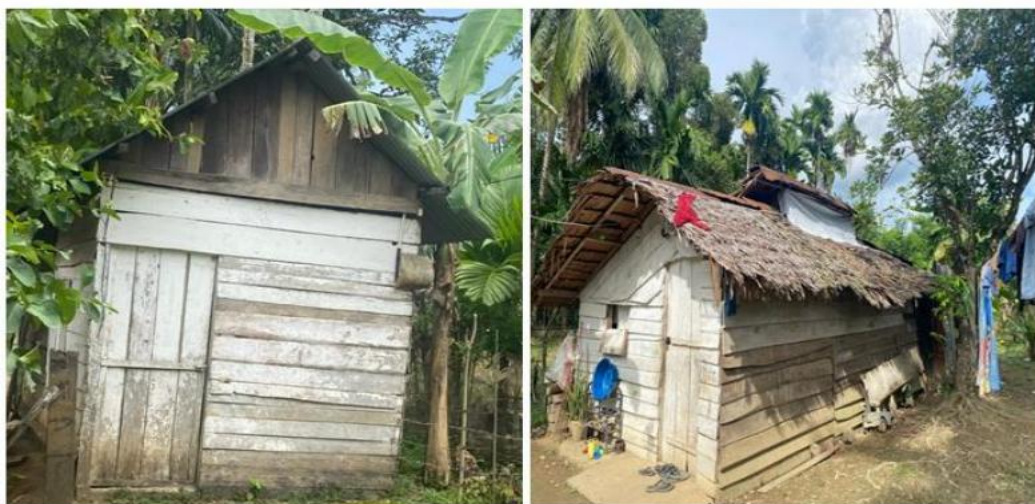
Figure 1.1. Uninhabitable Houses in Pantan Reu District
